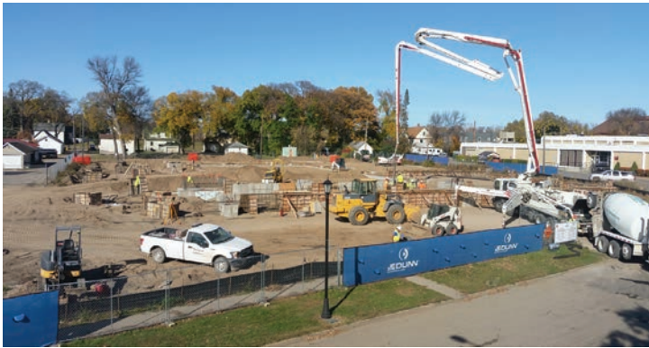
A recent webcam screenshot shows construction progress on the new Center for the Arts.
