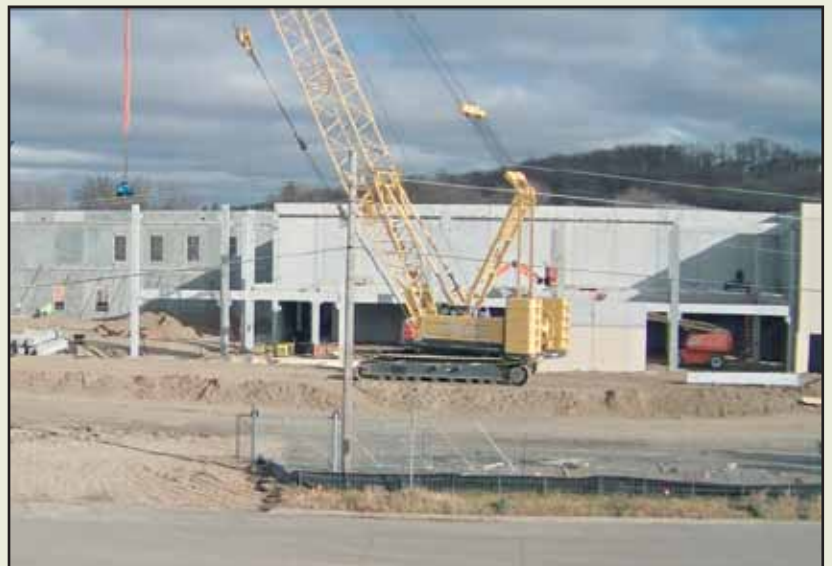
A large crane has been setting the precast wall panels in place at the Wellness Center. View construction progress via a webcam at technologyservices.vcsu.edu/vp.htm?p=3420 .
